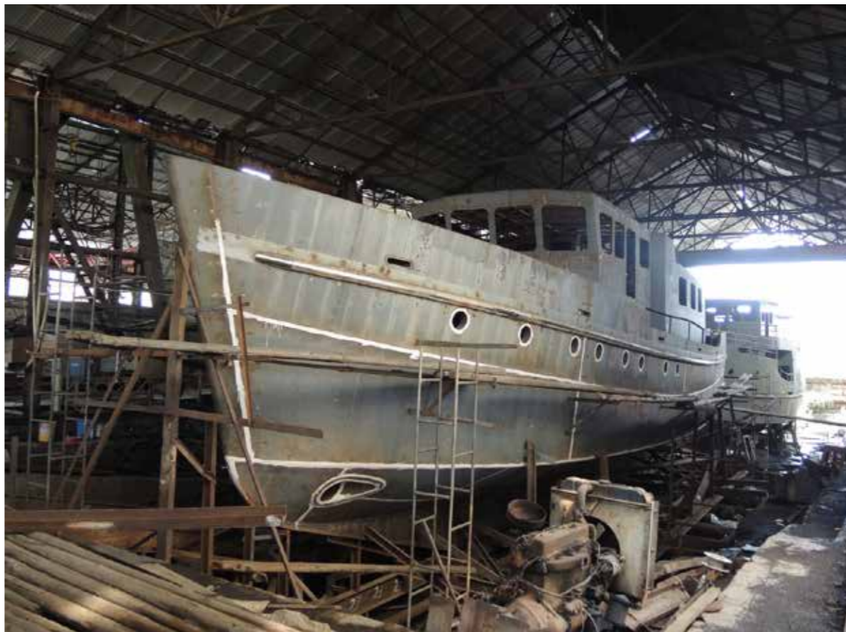
Above: Construction is a steel hull, deck, and pilohouse with fiberglass fly-bridge.
